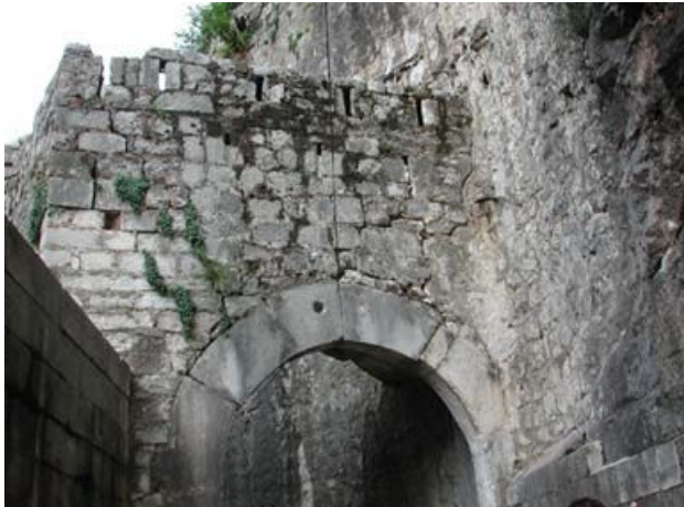
Defective crenulation and cracks.
